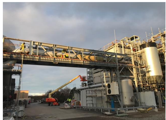
Insulation of flue gas pipes
