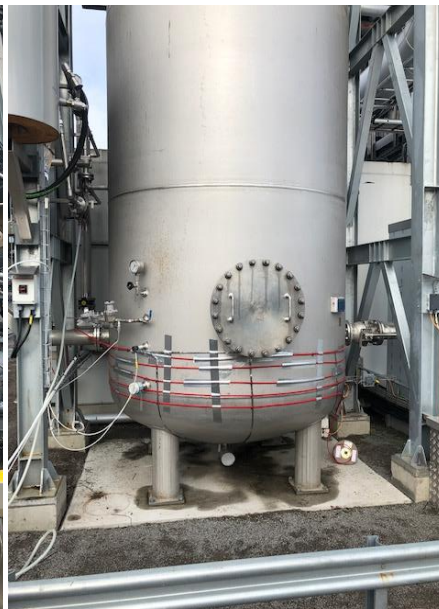
Expansions vessel after the syngas compressors.
