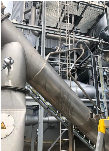
Outlet screw from pyrolysis during ongoing cold tests.
