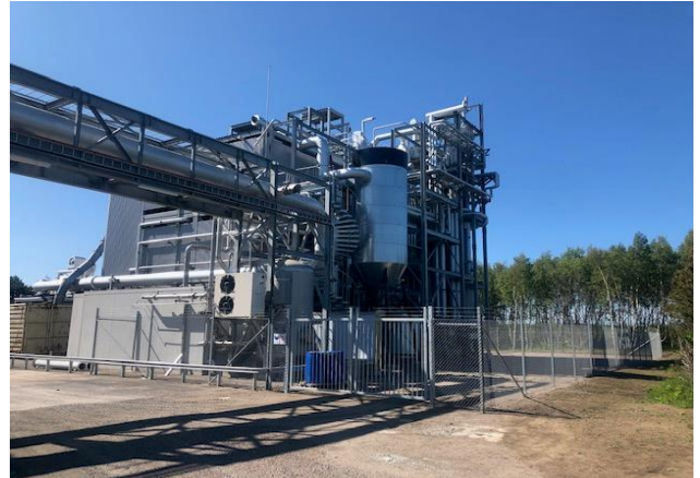
In the background one can see the filter and the steam system
