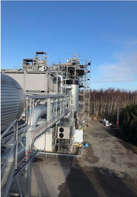
Sunny morning where the filter system is seen in the background
