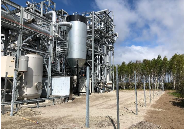
Construction of fence was started in April and completed during early May.
